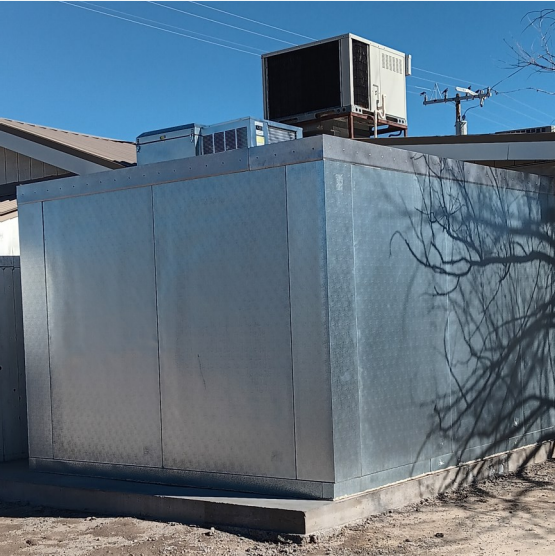
Refrigeration Unit for Willcox Community Food Pantry
