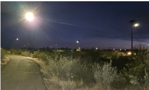
Airport Park walking path solar LED lighting
